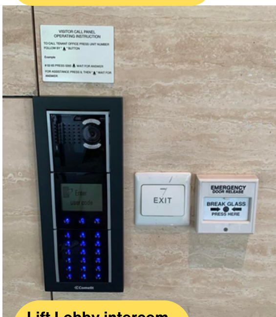
Lift Lobby intercom, press 0252
